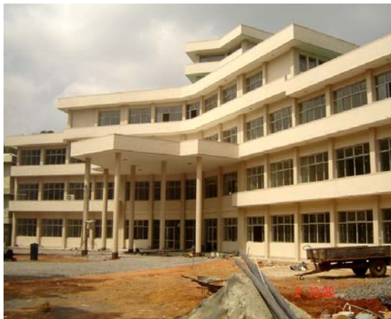
Four storied OPD and clinic complex at General Hospital – Vaunia under the NECORD Extension Project
