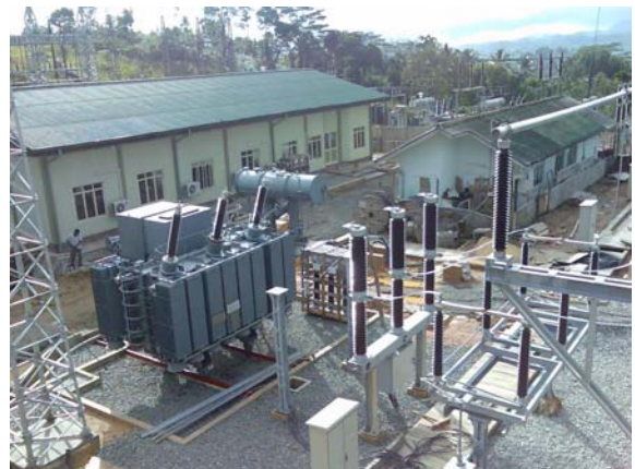
Deniyaya Grid Substation
