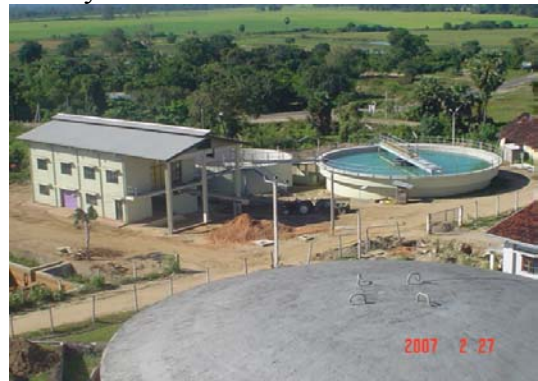
Centrifuge building at Treatment Plant Konduwatuwana
